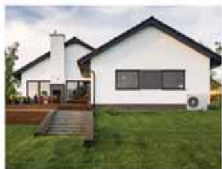
Air Source Heating
